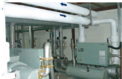
Machine Room for Conventional Central Water-source Unit
